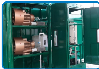
SEWAGE TREATMENT PLANT(STP)
