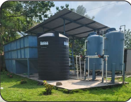
SEWAGE TREATMENT PLANT
