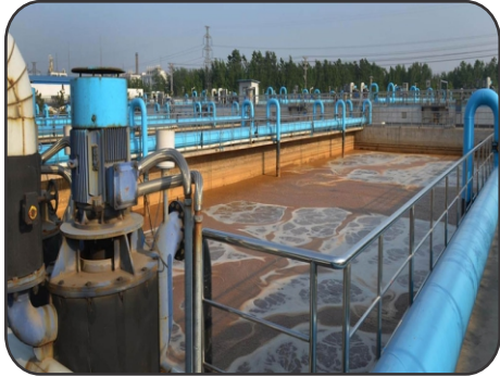
EFFLUENT TREATMENT PLANT
